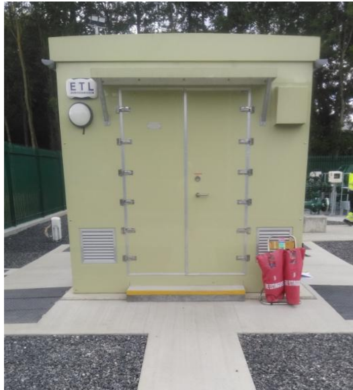
Figure 45: Typical E&I Kiosk
