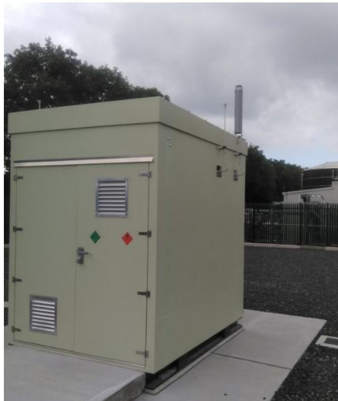
Figure 46: Typical Gas Analyser Kiosk
