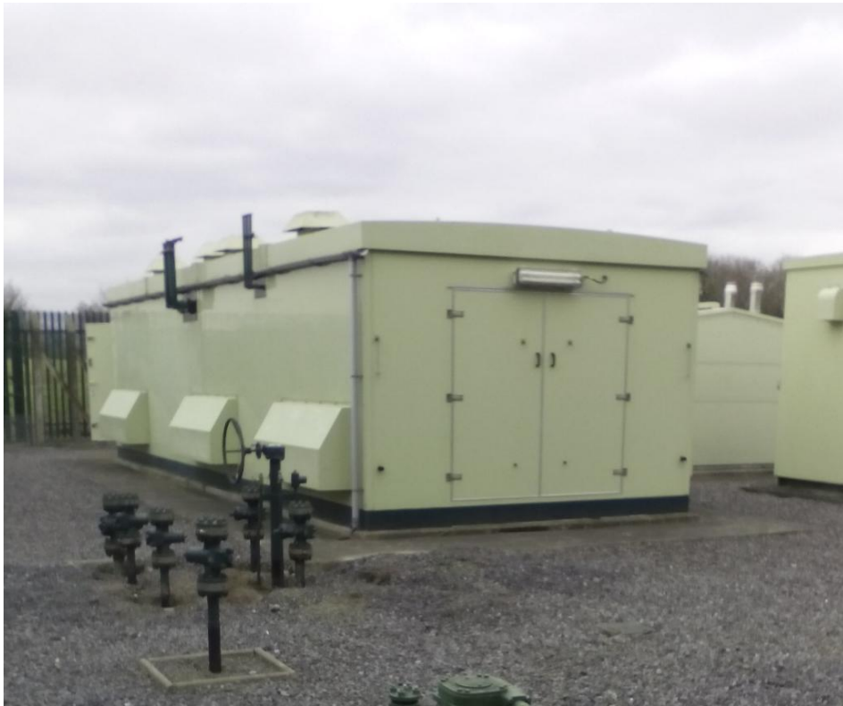
Figure 43: Typical PRS Kiosk
